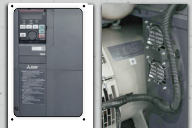
7 | 480V Variable Frequency Drive with Cooling Fans
