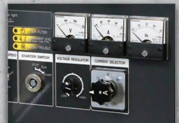
1 | Voltage Adjuster and Current Selector Controls
